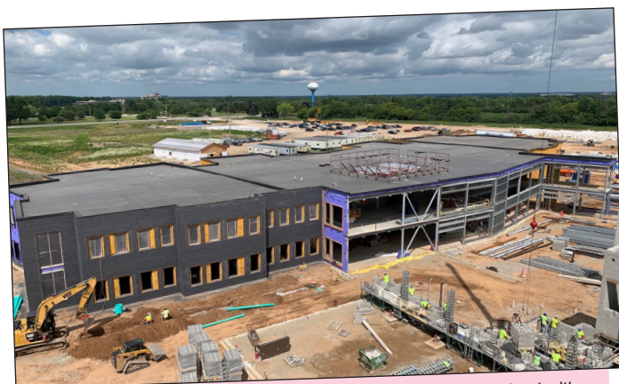
Construction is on schedule for the new Neenah High School with completion anticipated in July 2023. For more photos and details on the project, check out pages 4-5.
