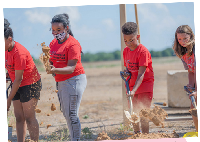
Future Neenah High School students were the first to put shovels into the ground for their new school on June 10 during the groundbreaking ceremony for the new Neenah High School that will open in the fall of 2023. For more information on the progress of the construction and other referendum projects, see page 5.
