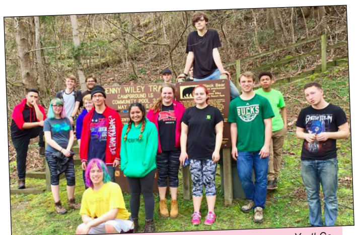
A group of 12 Neenah High School students were among a YouthGo team that worked on six homes for the elderly in rural Kentucky over spring break. Jobs consisted of building ramps for those in wheelchairs as well as replacing windows and doors on homes.
